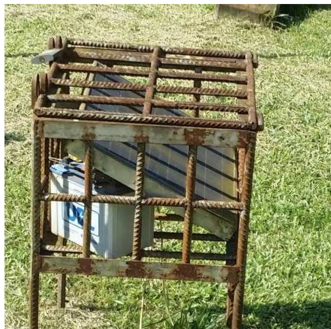
Figure 6 Securing solar panels and batteries using cages is common in East Africa
